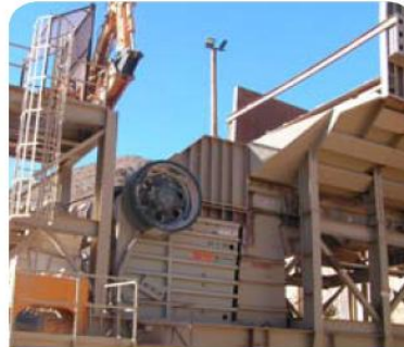
Aggregate Plant Boulder City, Nevada
